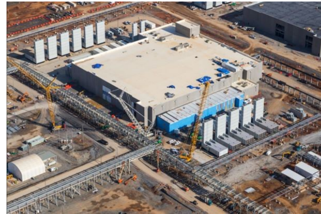
Google Datacenter, USc
