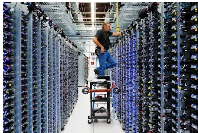
Inside the Google Datacenter
